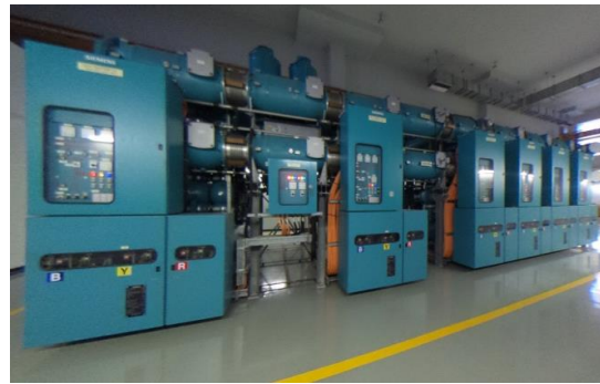
Gas Insolated substation
