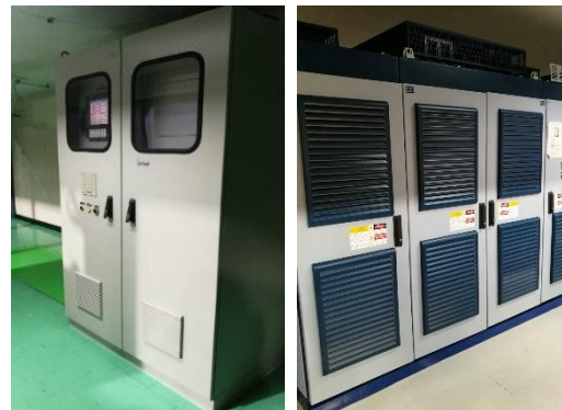
Variable Speed Drive
